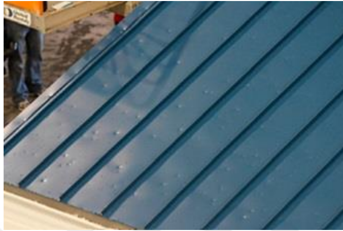
Figure 2. An example of a roof panel that has been damaged by hail Source: https://royalroofinginc.com/
