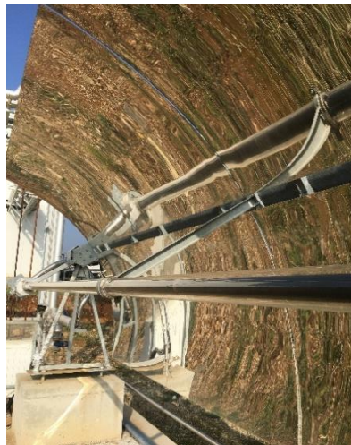
Figure 3.20. Support bracket of HCE at ADU Solar Field
