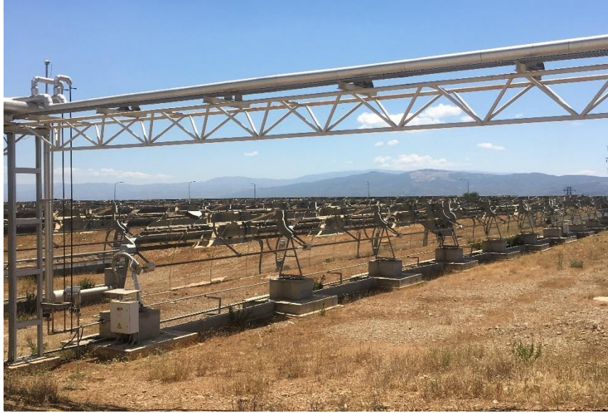
Figure 3.14. ADU Solar Field
