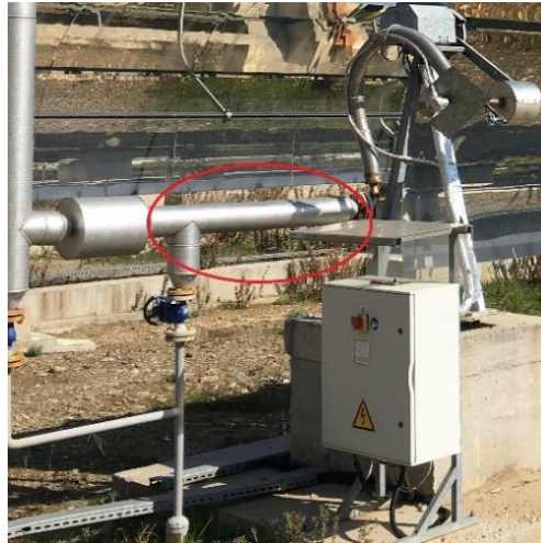
Figure 3.24. Other pipe next to the horizontal pipe
