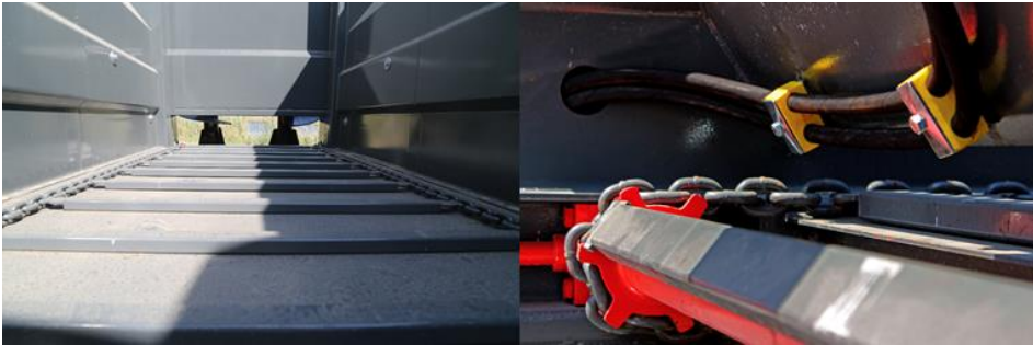
Figure 3.4. Conveyor mechanism inside trailer
