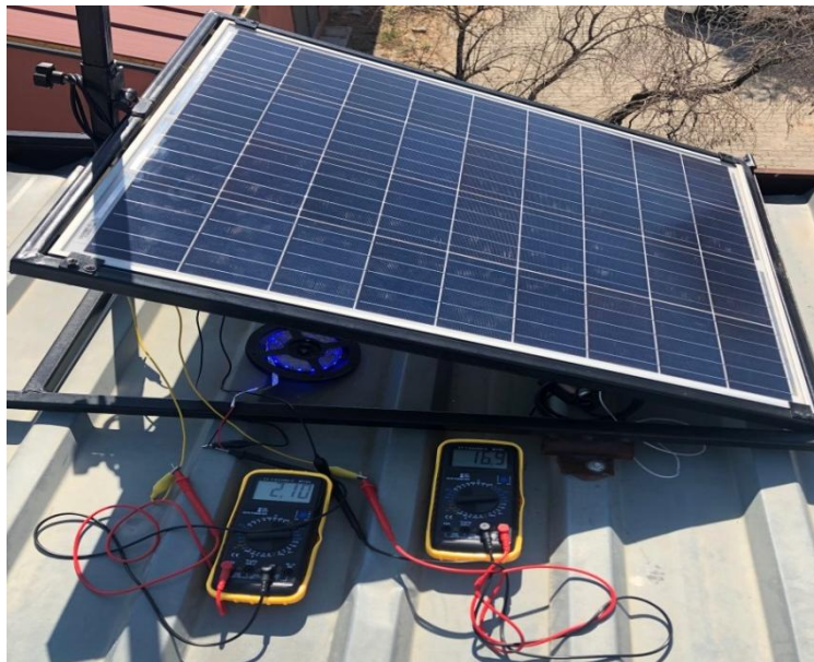
Figure 3.2. Polycrystalline photovoltaic solar panel
