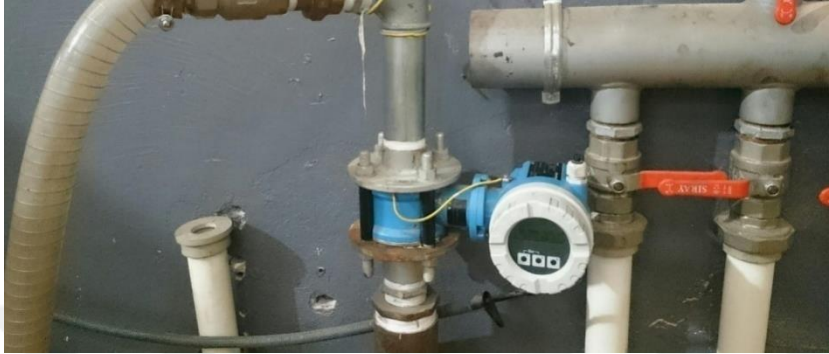
Figure 3.14: A photograph of the flowmeter.
