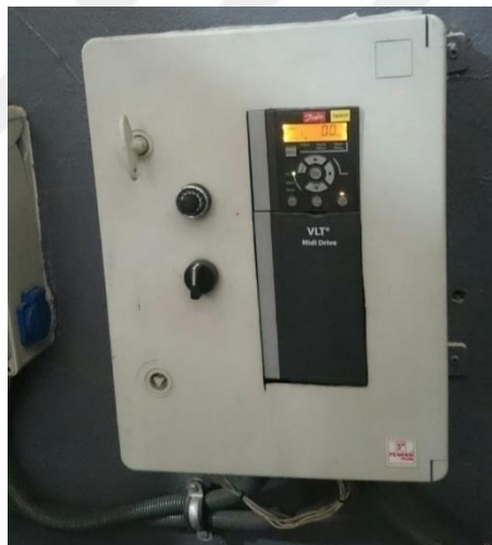
Figure 3.13: The VFD of the feed pump.
