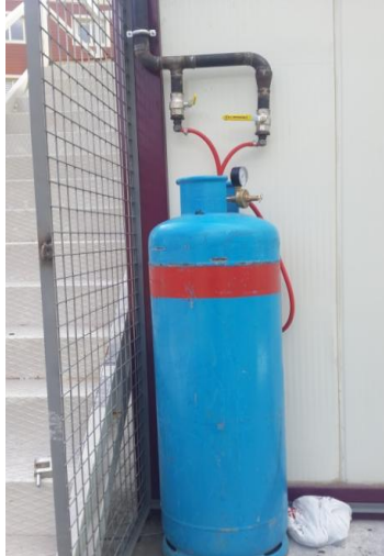
Figure 3.24. Gas Supply Installation with gas tube
