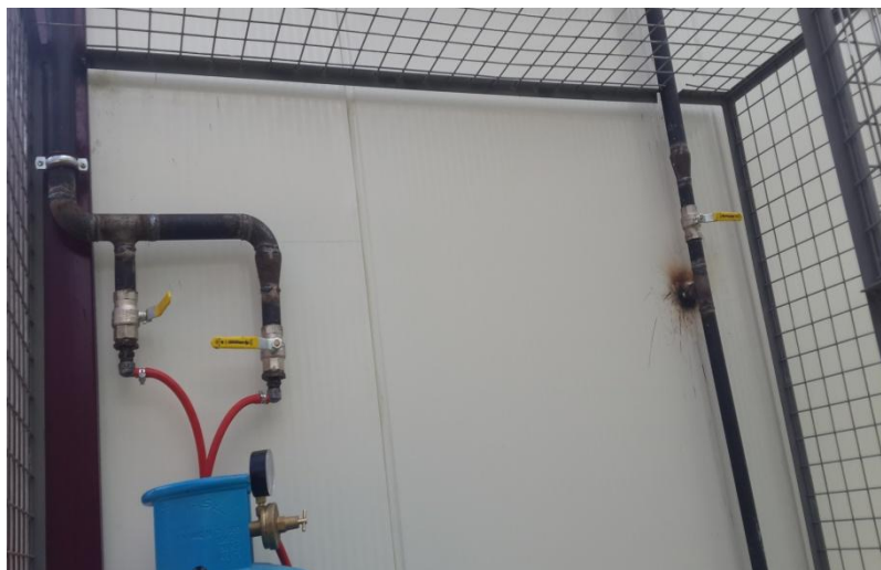
Figure 3.25. Gas supply Installation
